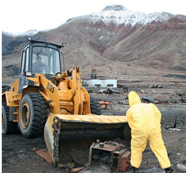
Leaking electrical equipment has been removed. From the removal work in Pyramiden. Photo: Halvard R. Pedersen
